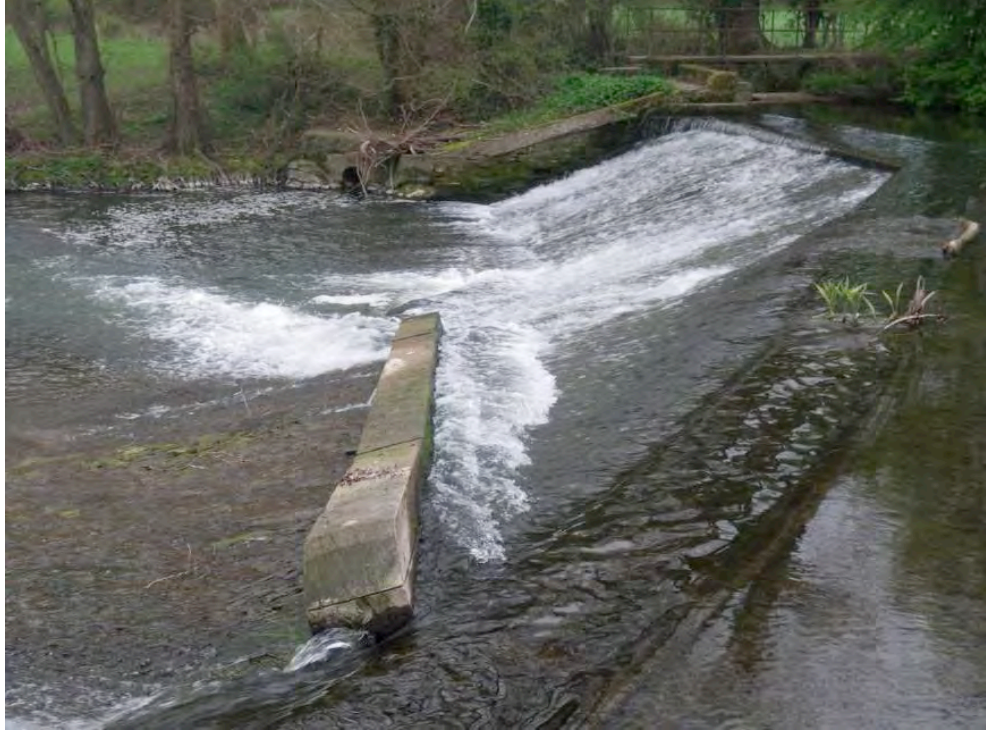
Figure 4: Baulk easement installed by the Wye and Usk Foundation. Sleepers are attached to the face of the weir by means of expansion bolts drilled into placements within the stonework (see Appendix 1 for E.A. guidance)
